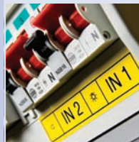
Distribution boxes & patch panels
